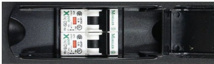
UL 489 hydraulic-magnetic circuit breaker on 30 Amp PDU.
