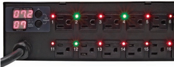
Rear of 2U PDU showing current draw for outlet #7. Red LEDs show outlets that are switched on. Green LEDs show outlets that are switched off.
