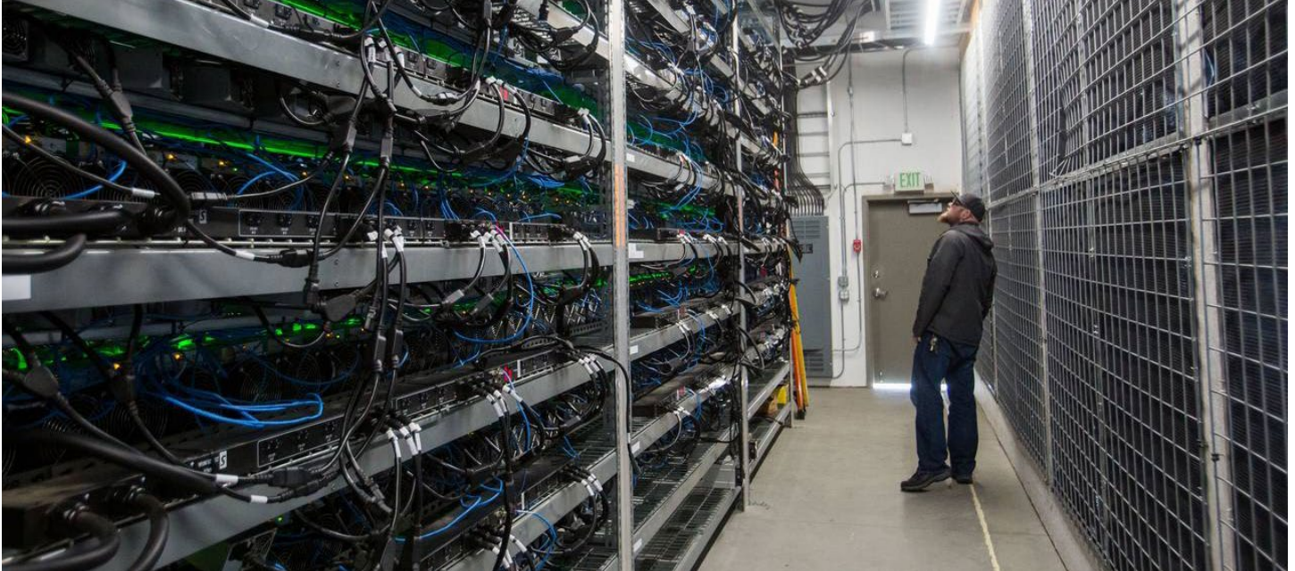
High density Raritan PX2 PDUs with dual inlet and 10kAIC circuit breaker per outlet with metering and switching, deployed in a high density crypto-mining facility in the United States.
