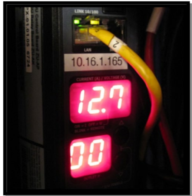
Figure 2. Raritan Dominion PX DPXS20A-30L6 deployed in J.R. Simplot’s data center showing rack loads.
